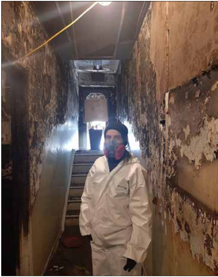
Ellen Millar inspecting fire damage at St. Andrew's Presbyterian Church in Barrie, Ont.
